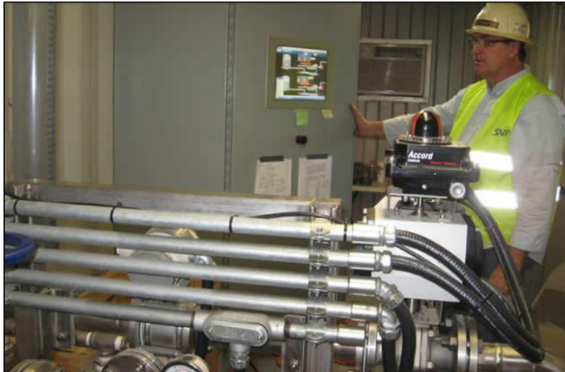
Figure 2: Polymer Preparation Plant (photo by Bankers Petroleum)
